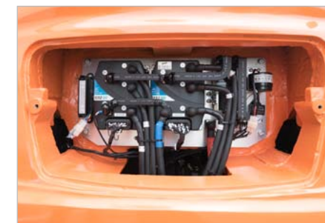
Easy to access controller room
